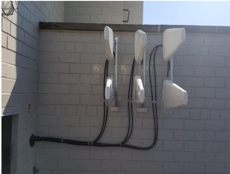
Exterior Antenna Array Deployment
